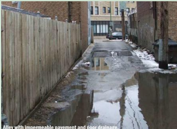
Alley with impermeable pavement and poor drainage.
