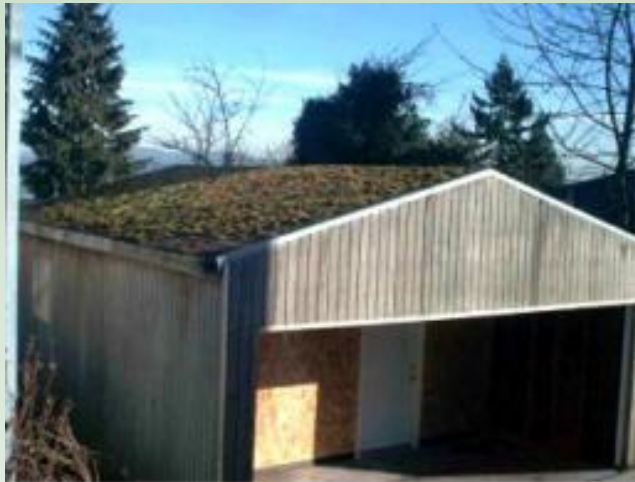
Neglected Garage – Nature Happens Photo Courtesy of Patrick Carey
